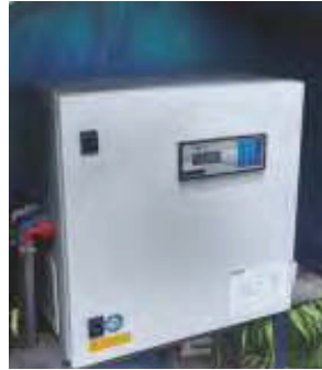
STP Compressor Panel & Water Treatment Plant
